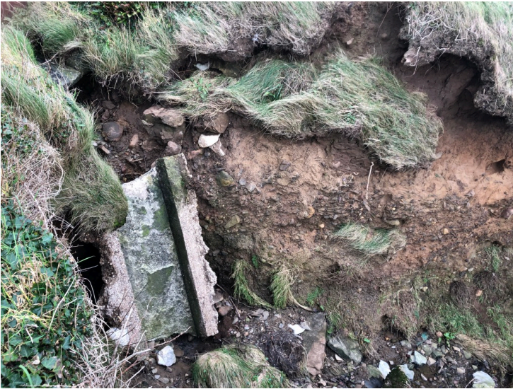
Photograph 1 - Existing erosion at SSSI, important for its Geological properties
